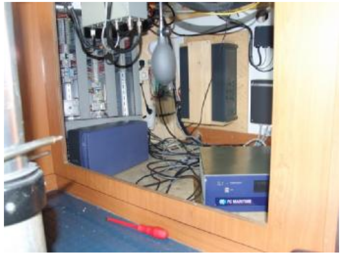
Figure 5 Boxes and wiring
